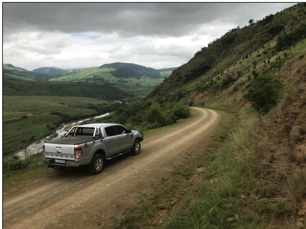
Figure 5-3: The Existing D1212 Road that needs to be widened with expected stabilisation of the cutting on the right
